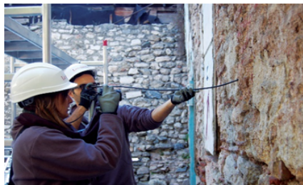
Figure 4. Examination of the micro cracks with camera.
