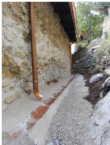
Figure 15. Away from the rainwater from the side wall
