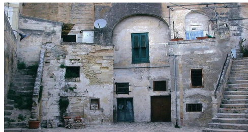
Figure 4: Degradation of the facades of the constructions overlooking the little square.
