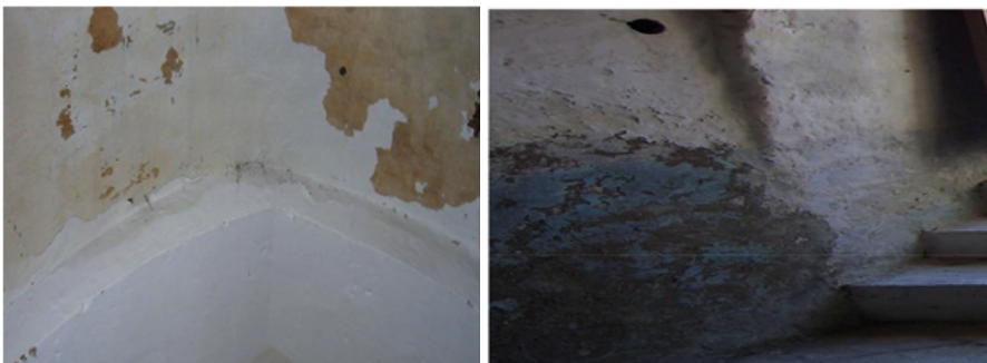
Figure 5. Decay of interior plaster based on organic polymers. Figure 6. Decay of interior plaster based on pigmented organic polymers.
