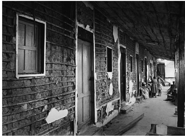
Figure 2. Bahareque building in El Salvador, after 1986 earthquake showing shedding of plaster from undamaged walls (6).
