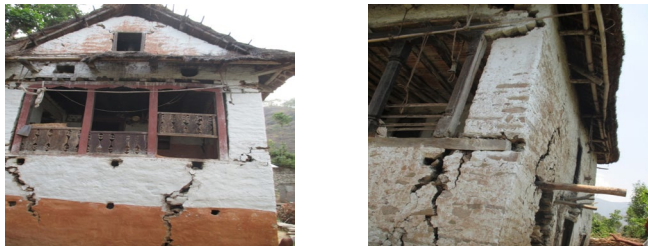
Figure 8. Typical large size opening in the side wall of the building, which causes large cracking in corner of opening
