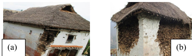
Figure 6. Observed typical connection failure at corner of wall (a) & (b) Delaminating of wall
