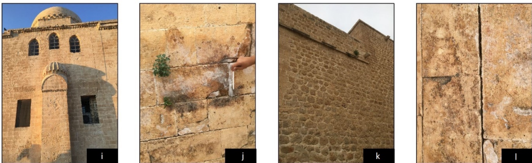
Figure 5. Biological distortions seen at Kasımiye Madrasa
