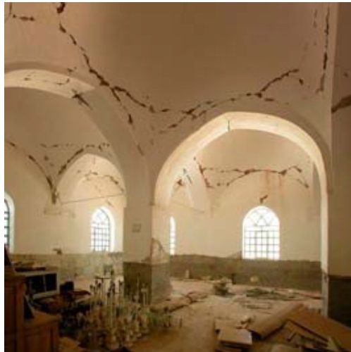
Figure 1. Interior of an adobe dome after the 2003 Bam earthquake, showing damage, but no collapse (3).
