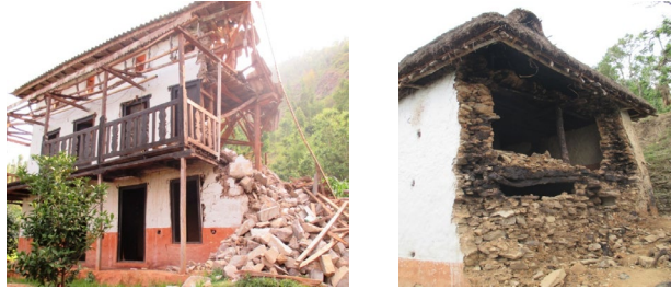
Figure 7. Totally collapsed building (left) & failed in out of plane (right)
