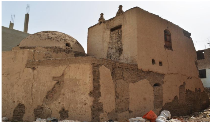
Figure 8. Wall Bulging and Slumping, El.Qurna- Luxor, Egypt, Taken by author
