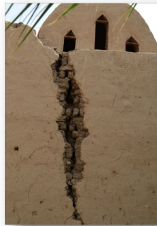
Figure 3. The cracks in a house wall, Qurna village- Hassan Fathi - Luxor – Egypt, Taken by the Author
