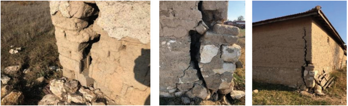
Figure 11 Workmanship errors at corner joints (2019).
