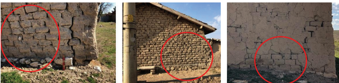
Figure 10 Traditional workmanship errors seen at adobe brick walls (2019).
