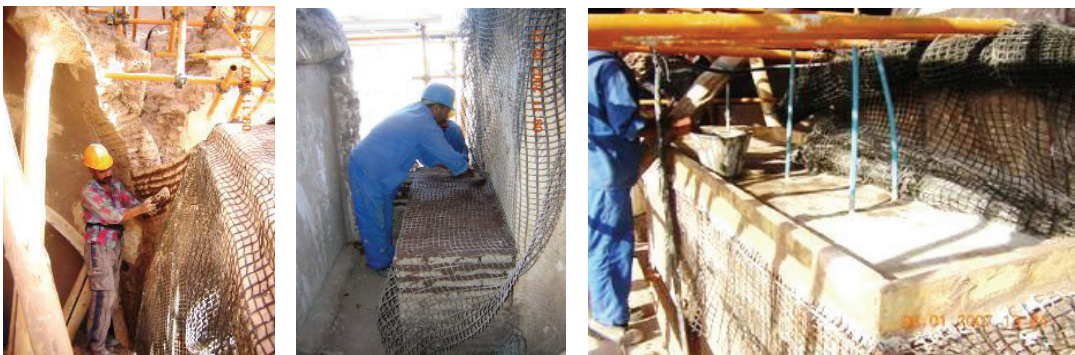
Figure 27,28,29 the bases are strengthen with plastic bars (Archives of bam's research center,1997).
