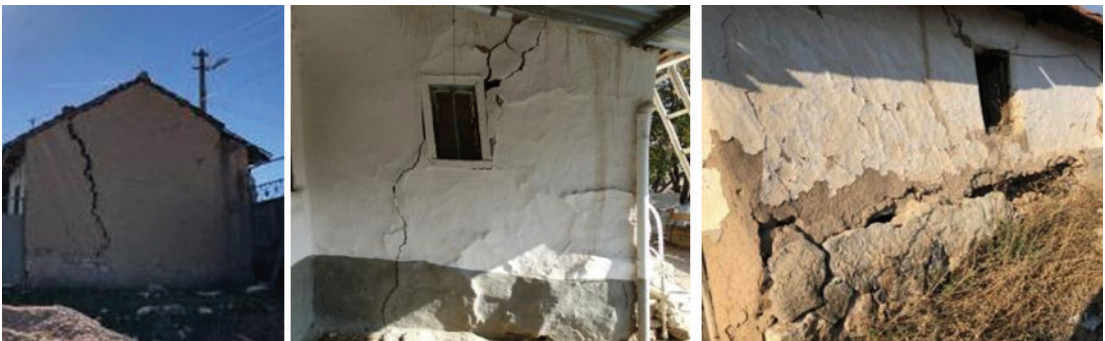
Figure 9 Earthquake structural cracks and lack of wooden tie beams (2018).
