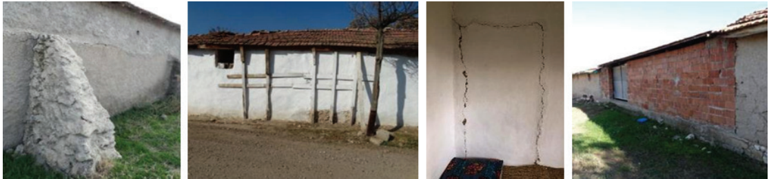
Figure 12 Unqualified wall repairs done with struts, metal belts and wooden elements (2018).
