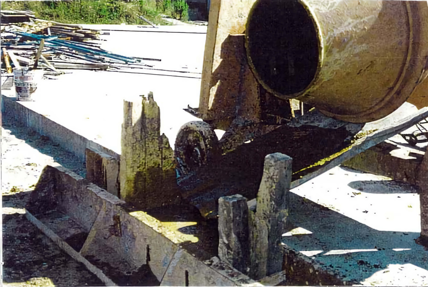
Resim 3.18. Likit Kıvamlı Harcın Kalıba Boşaltılması Picture 3.18. Discharge of Mortar at Liquid Consistency into the Mould
