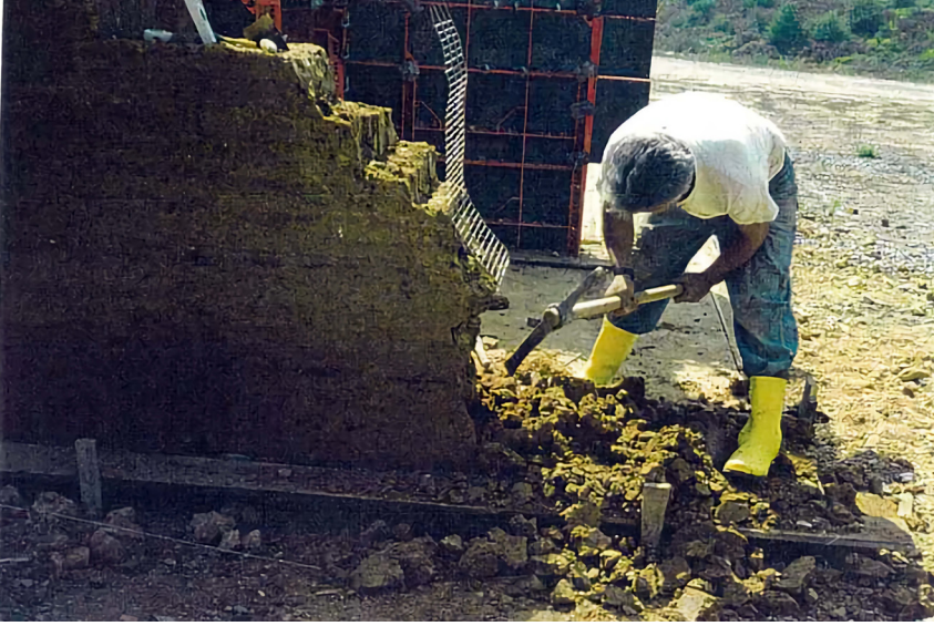
Resim 3.32. Duvar İine Yerleřtirilen Deprem Hatlı Picture 3.32. Tie Beam for Earthquake Placed into the Wall
