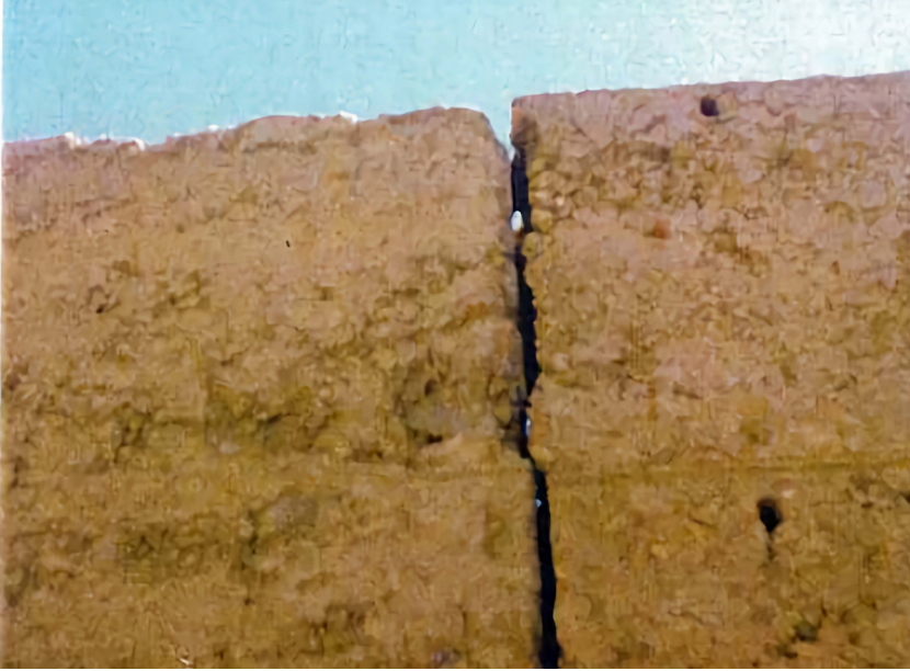
Resim 3.23. Farklı Zamanlarda Dökülen Duvarlardaki İş Derzi Problemi Picture 3.23. Problem regarding Construction Joint in Walls Casted at Different Times
